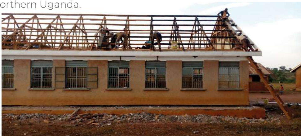
Reroofing a classroom block at Alao Primary School in Oyam District, Uganda. January 2022.
